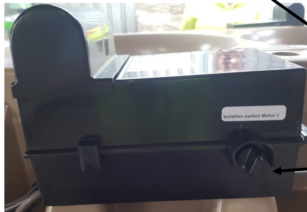
Motor No. 1 Isolation Switch
